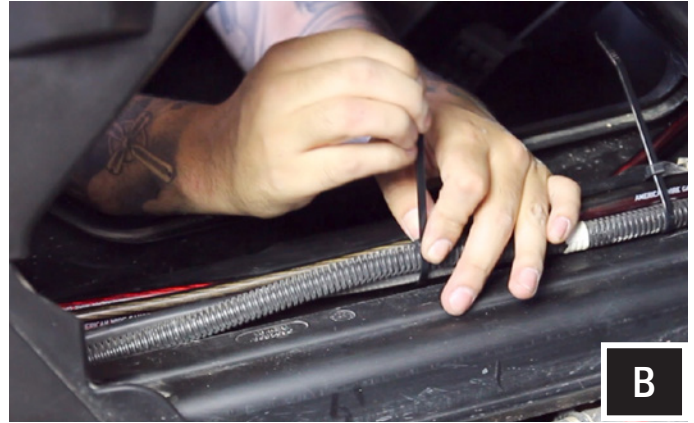
B. Zip tie all cables to the factory cabling along the center column away from the drive shaft.
