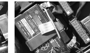
3. Once unfastened, connect the black harness cable to the negative battery terminal and tighten down to the manufacturer's specs.
