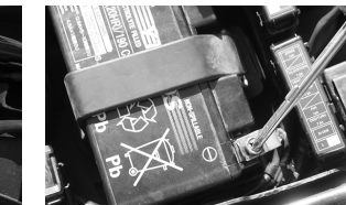
2. Using a 10mm wrench or screwdriver, loosen the bolts attached to the terminals. (Make sure not to touch both terminals at the same time)
