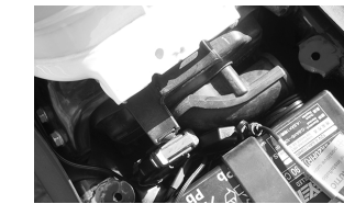
4. Connect the red cable to the positive terminal and tighten down to the manufacturer's specs.
